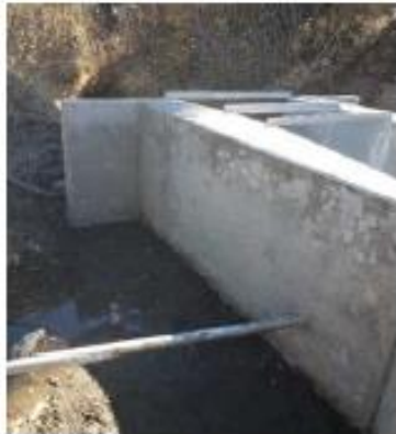
2" Sch 40 galvanized steel inlet pipe
