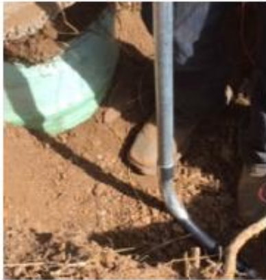
90 degree sweep at base of mast
