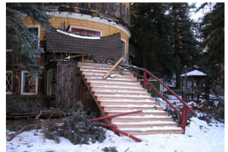
Fallen trees damaged the front porch at the historic Glen-Isle Lodge in November.
